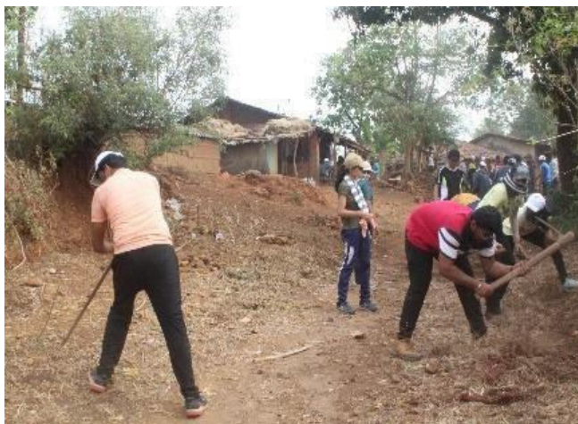
NAME OF THE ACTIVITY: Repairing of Raw Road (Sadak)& Creating a pathway to Farm at Adopted Village Palsunde DATE: 20th March 2022 to 26th March 2022 TIME: 10.00 AM TO 5.00 PM Venue: Palsunde, Mokhada
